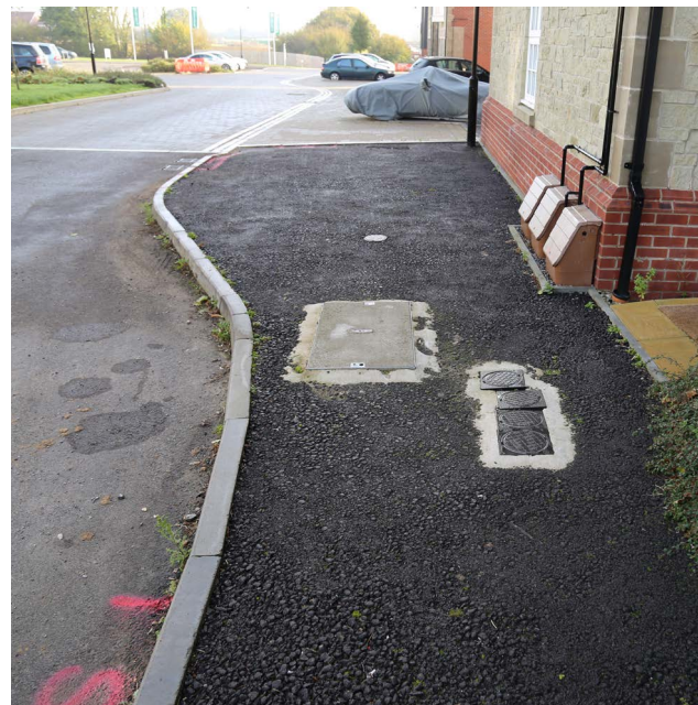
Poor quality road surface, Mampitts Lane
