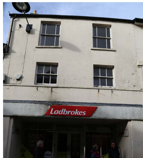
Poor quality shopfront High Street
