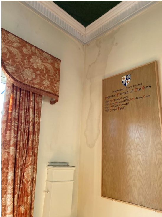
26: Staining to the SW corner of the chamber
