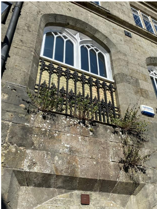
18: painted brickwork railings and vegetation
