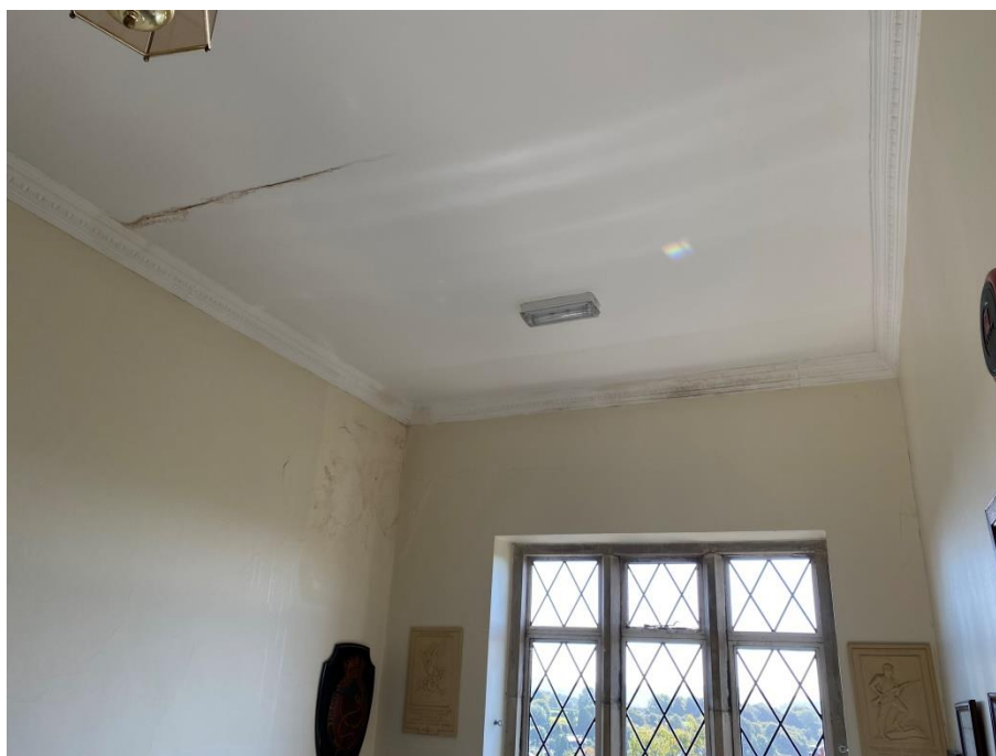
28: Stains and cracks to ceiling over stair case, and landing (including stains to cornice)
