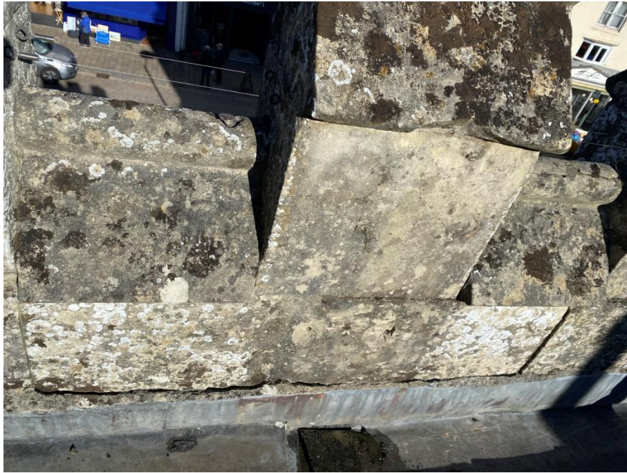
12: Stone block to parapet out of place (where flagpole previously fitted)
