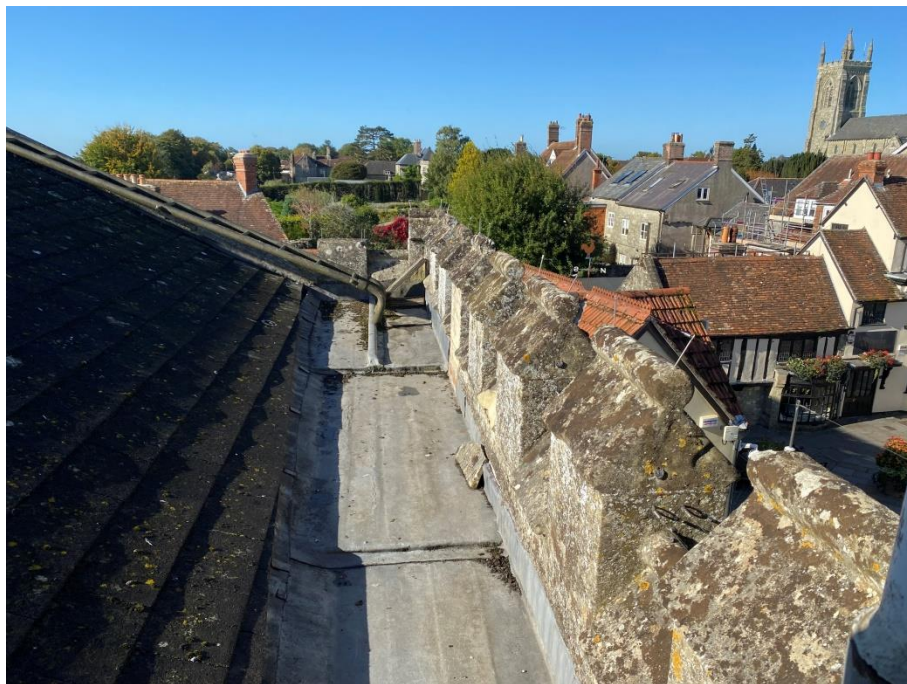
3: North West lead lined gutter, fractured stone (RHS) missing merlon
