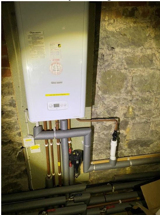
7: Boiler within roof space – uninsulated pipes
