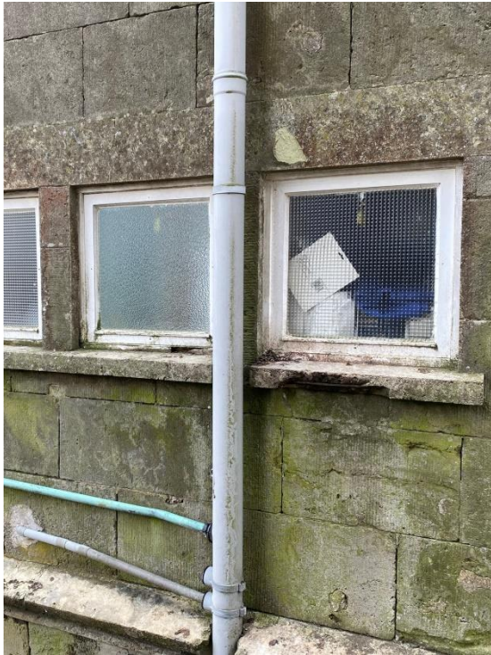
22: Blown window cill to w.c.s
