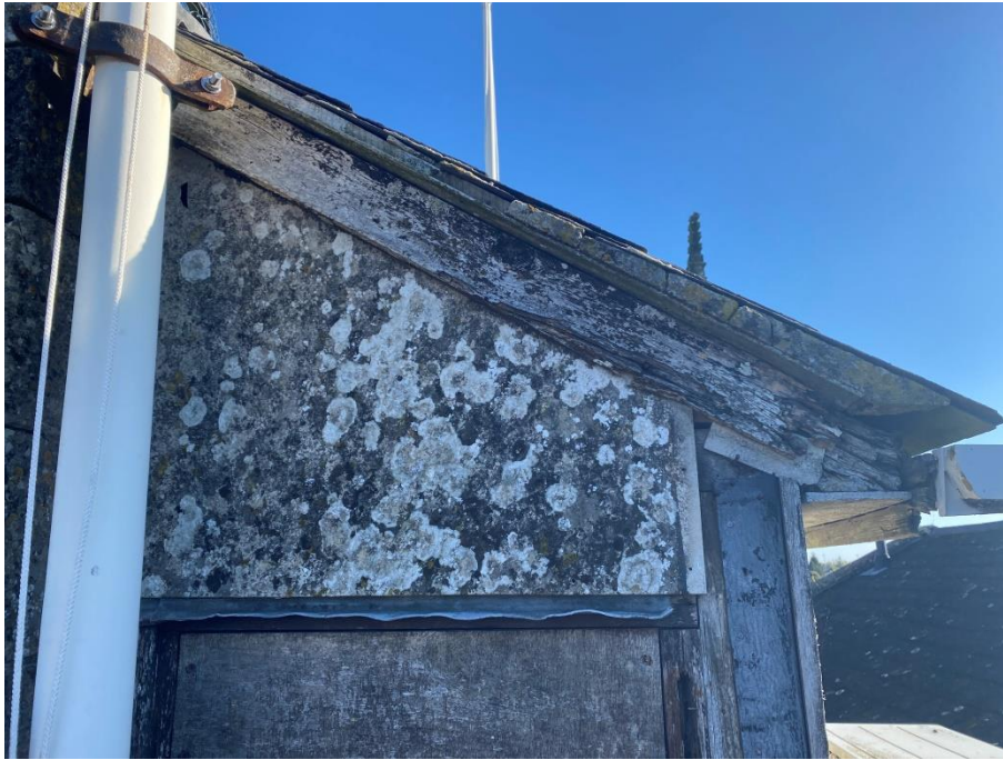
4: Asbestos clad clock room, rotten barge boards, missing cover board
