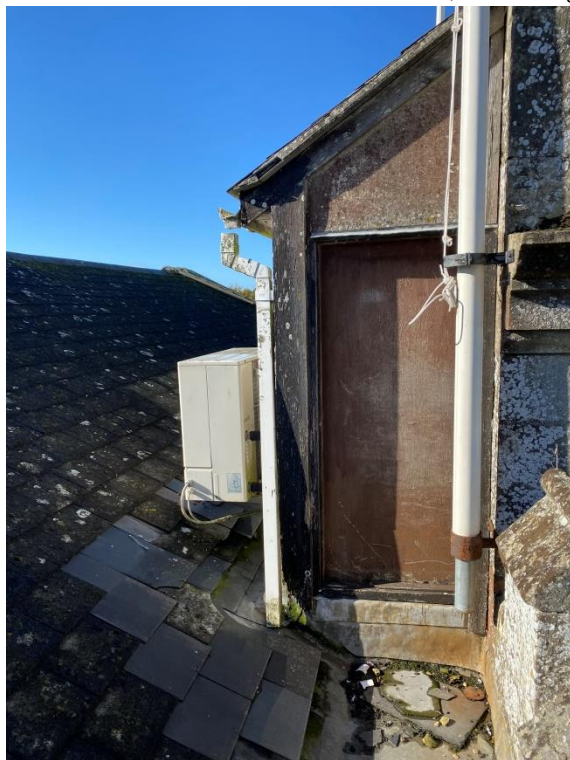
5: Ply door to clock room, replaced/broken slates, gutter remote from downpipe.
