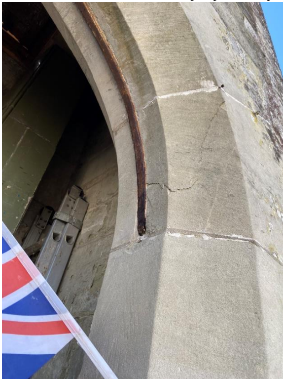
13: Corroded strap beneath clock tower arch
