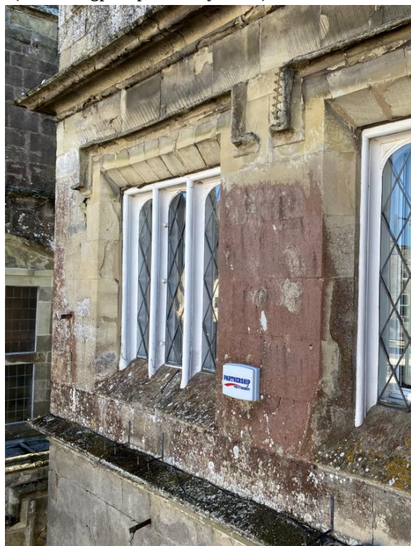
14: North East corner scaling and previous mortar repairs
