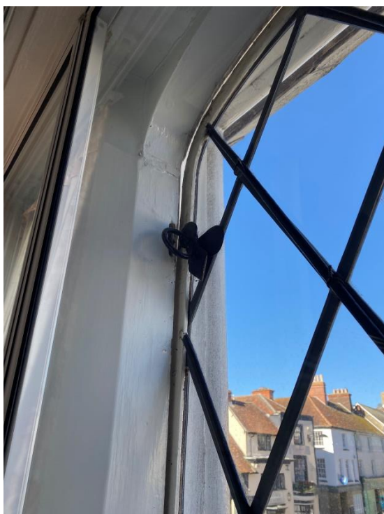
24: Ill-fitting leaded casements to North windows
