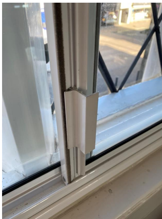
25: Incorrectly assembled secondary glazing.
