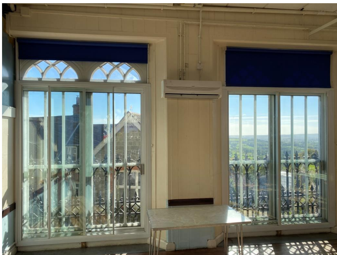
30: Barrier to the views by railings, timber frame, patio doors and secondary glazing
