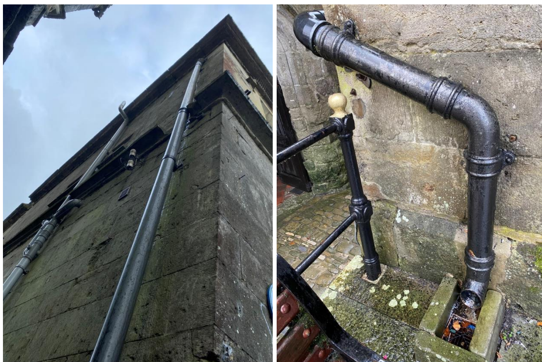
10: Plastic downpipe to NW corner wall damp behind 11: Last cast iron section and shoe into gully
